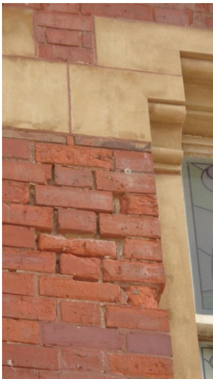
Late Victorian building repointed with cement mortar which has led to frost damage
