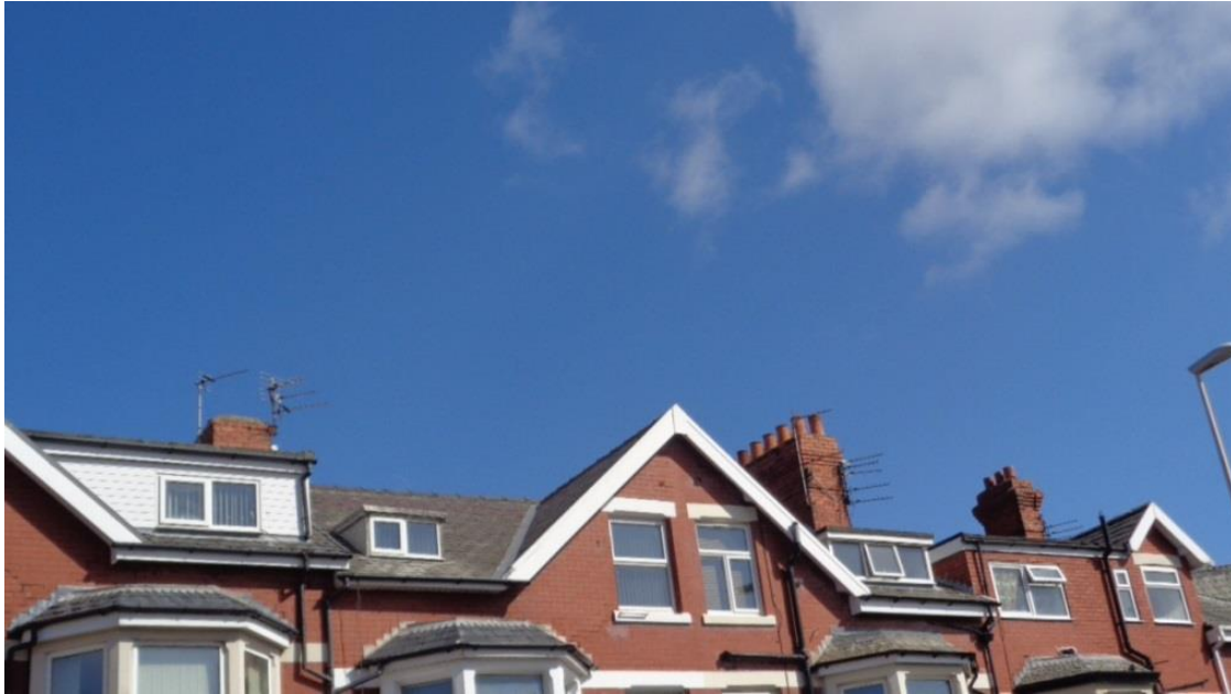
Differently designed roof lifts on a single terrace
