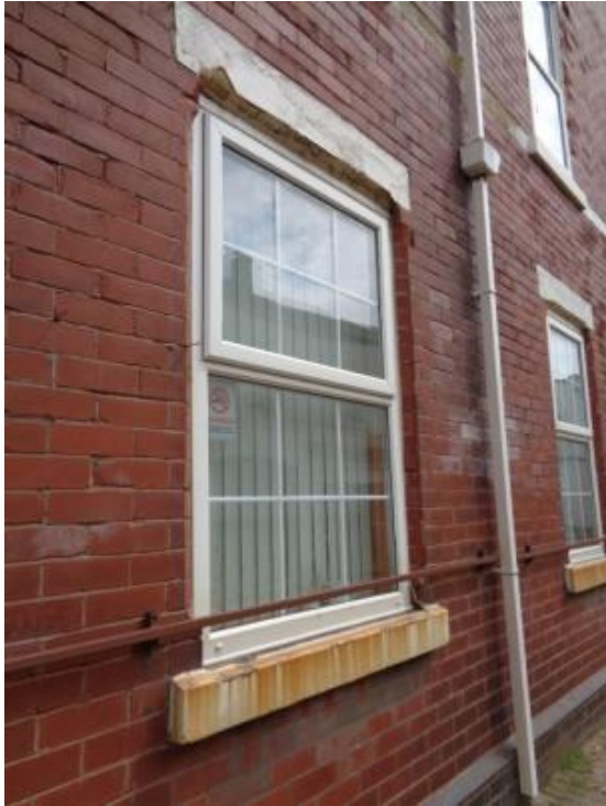
Upvc window frame with 'stick on' glazing bars and top hung upper window
